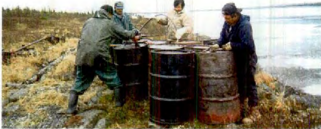
Photo 6. Transfer of waste liquid from barrels using a pump at Site 224A (June 26, 2000). Water constituted more than 90% of the waste liquid.
