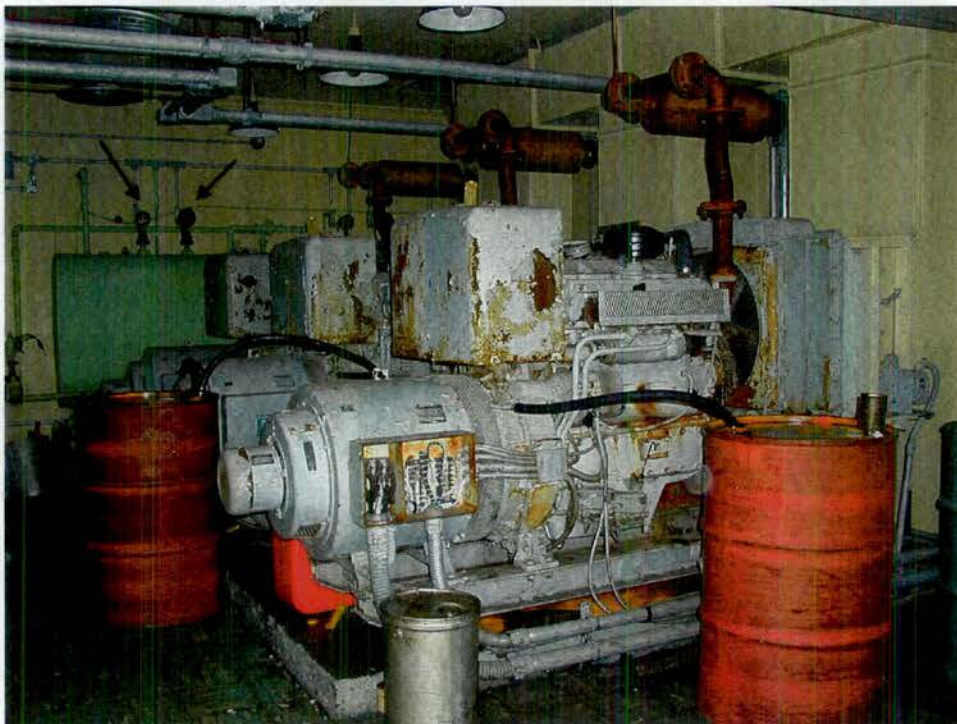
Photo 2. Draining generator oil tanks at Site 321 (September 8, 2000). Note: round metal boxes (arrows) on one of the tanks located at the end of the room contain mercury switches.
